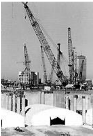
"Tunnel Vents with Hancock Tower": A Photo of Boston's Big Dig ©Miriam Goodman.
